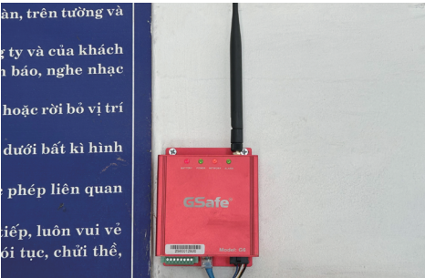
Fire Alarm Transmission System (SeAH Steel Vina)
